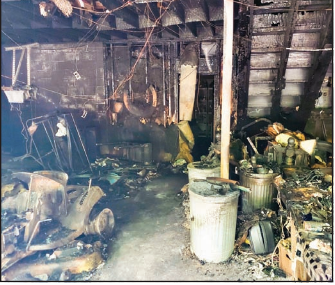
Anyone with info regarding this basement fire at 1500 Sunnyside Road should contact Fire Chief Harold Copeland at 706-994-4934 for a potential reward. Photo/Submitted
